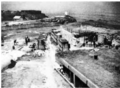
View from the Battery Observation Post (BOP) of the construction of the underground magazine and 6-inch gun emplacement (Gun No. 2). In the background can be seen the remains of the Portuguese Fort St Joseph. Photo: The National Archives, Kew.
